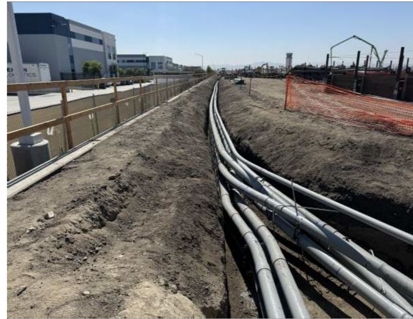
East Retaining Wall Ductbank
